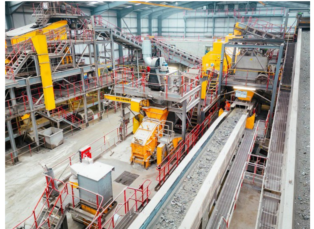
IBA PROCESSING FACILITY, FERRYBRIDGE, UK
