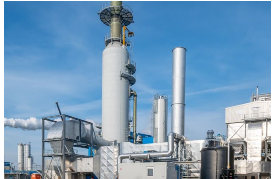
THERMAL TREATMENT GASIFIER, NETHERLANDS
