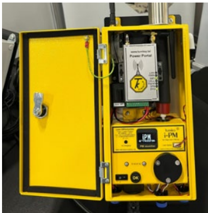
ADVANCED DUST MONITORING EQUIPMENT AT OUR SITE BOUNDARY IN SHEFFIELD
